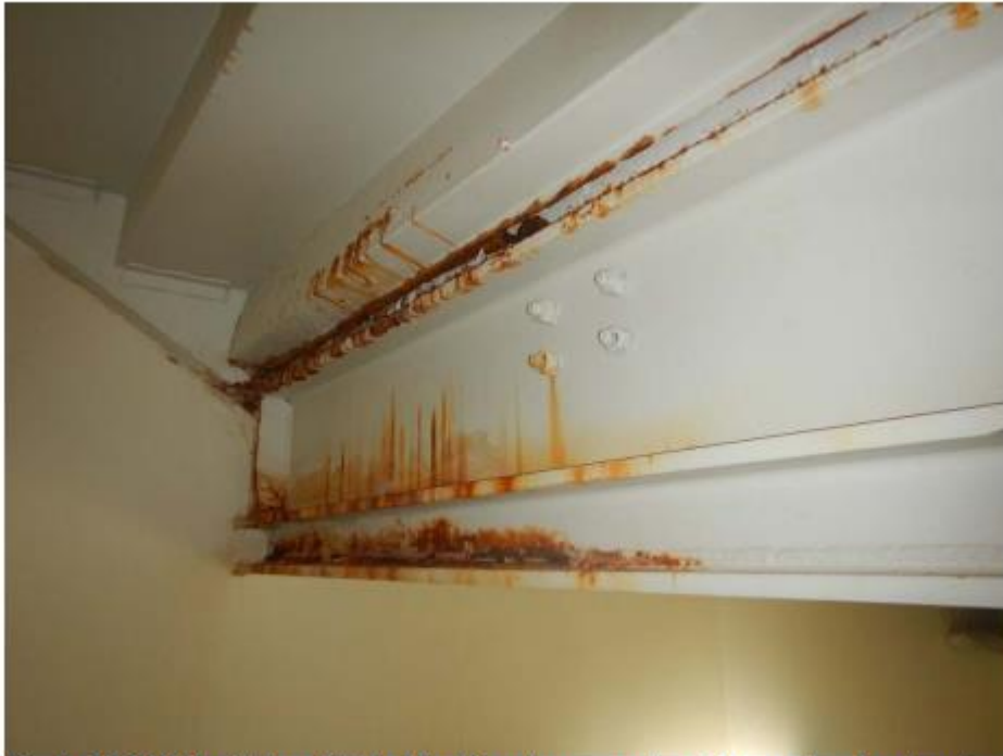
Photo 12(2021) – Stairwell 5 landing framing corrosion at lower landing levels.
