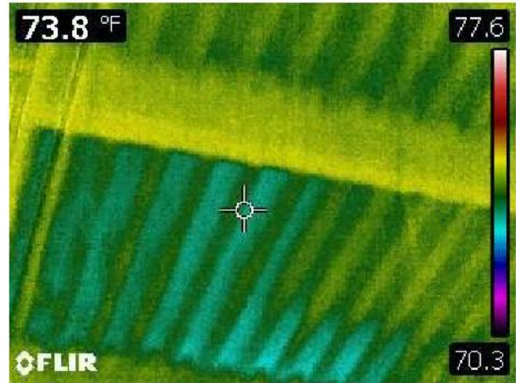
Photo 18: An infrared image of the area depicted in Photo 17 shows the moisture above the slab or the underlying fireproofing in this location of Storage Room 339.
