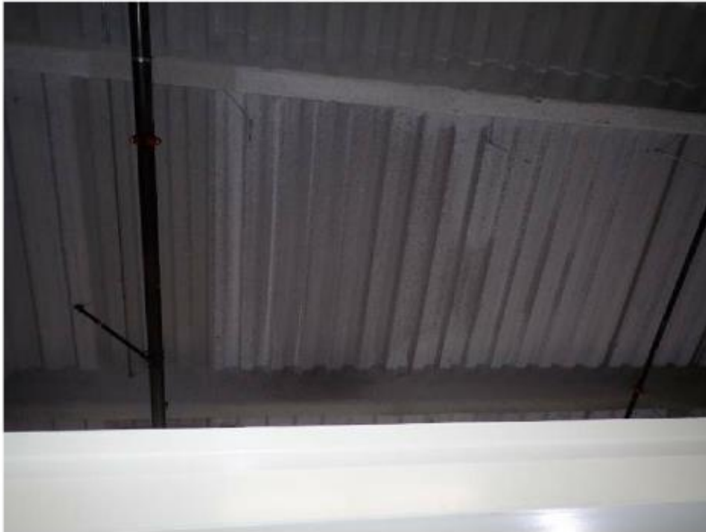
Photo 17: An observable dark area of fireproofing is located at the ceiling of Storage Room 339. Please refer to the infrared image in Photo 17 to view the moisture above the metal decking in this area.
