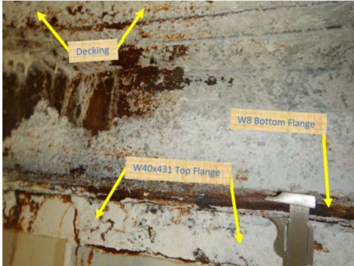
Photo 8(2021) – Ewa end of Stairwell 5 at corroded W8 (GL H) and decking atop W40x431.
