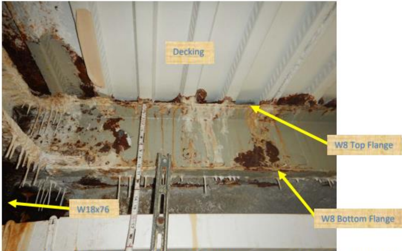
Photo 10(2021) – Diamond head end of Stairwell 6 at corroded W8 (GL I) & decking over W18x76.
