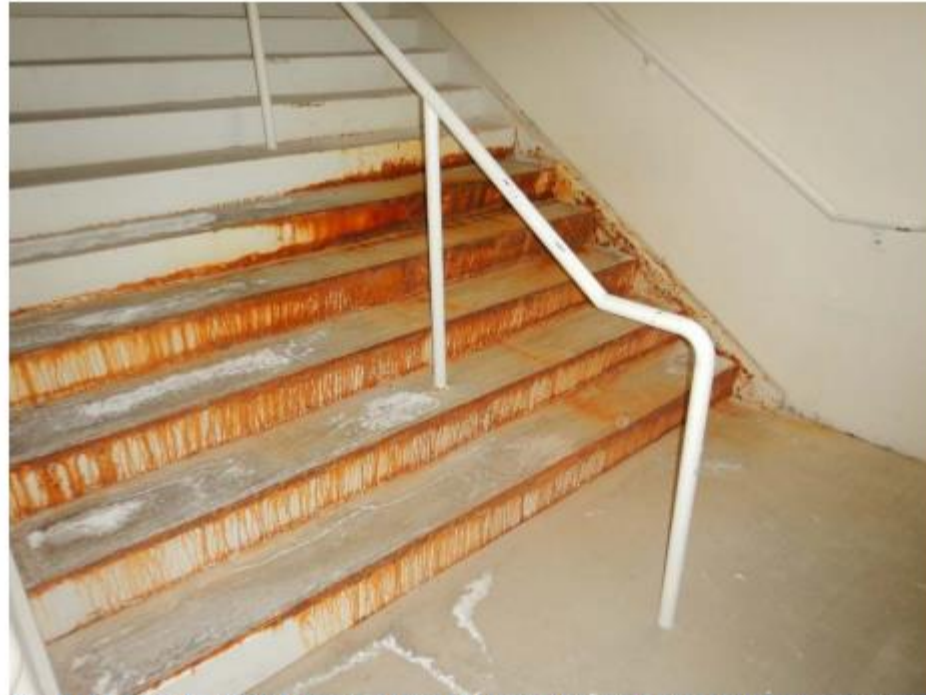
Photo 13(2021) – Stairwell 5 step pans and landing framing corrosion at lower landing levels(1of2). Temporary shoring below is recommended. Suggest sealing stairs water tight, remove surface rust, and coat.
