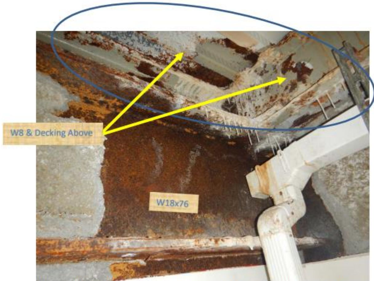
Photo 9(2021) – Diamond head end of Stairwell 6 (intersection of GL 3.4/l) at corroded W18x76.
