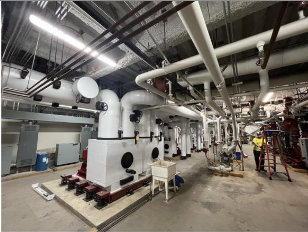
New LED lighting enhances the new chiller equipment. HCC hosted Green Business executives attending the National Summit in Honolulu for a site visit of our new sustainable chiller system.
